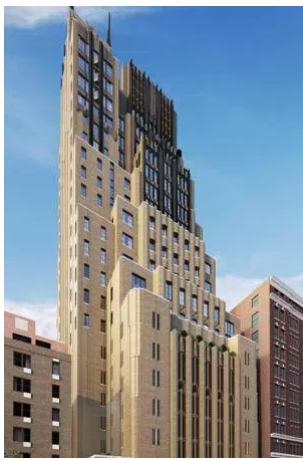
A 1929 Art Deco classic is being converted into Walker Tower, with 53 condo units under construction. ( )
